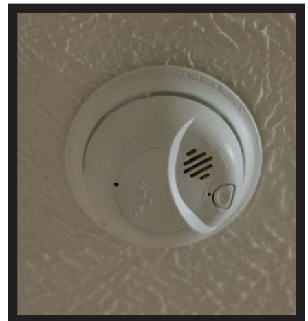
Smoke Detector Carbon Dioxide Detector
